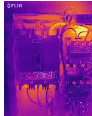
Identify electrical faults
